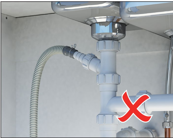
Incorrect waste pipe configuration.
