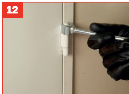
Gap between the door edge and the frame should be between 2-4mm. Adjustments can be made using a cranking tool. To ease the door leaf towards or away from the jamb, apply slight pressure to the tops and bottoms of each hinge knuckle. Ensure that a consistent gap is achieved all around the door. Ensure all packers are pushed up into the gaps.
