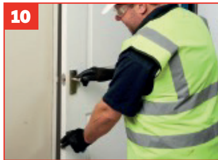
Test the door closes in the frame correctly, ensuring that the door does not bind or catch
