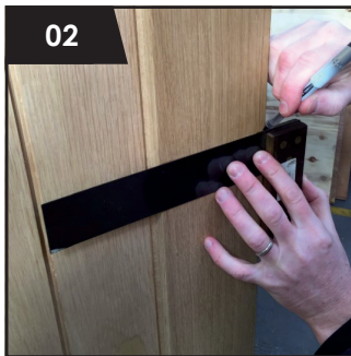
Measure and mark the door handle height. 1.0 metre from floor level is typical.
