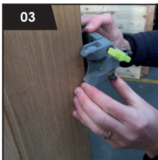
Adjust the backset to suit tubular latch specification – 45mm or 57mm. Remove the reducing sleeve for Jigtech latches. Align the jig with the height mark. Clamp the jig to the door securely without over tightening.
